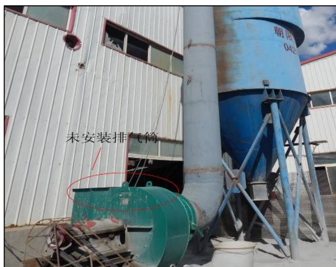
除尘器排放口不规范
